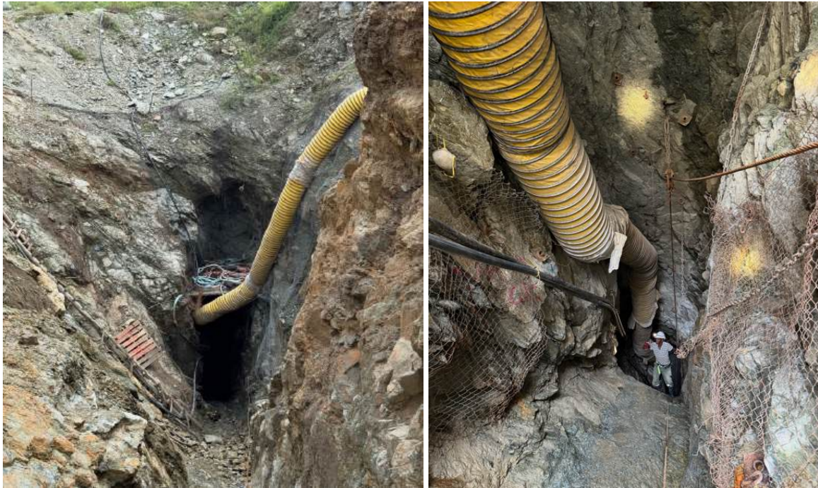
Figure 4: Ventilation in winze
