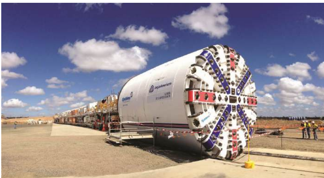
Figure 10: A Robbins Dual Mode EPB/Rock TBM Grosvenor Decline Tunnel Project in Queensland, Australia.
