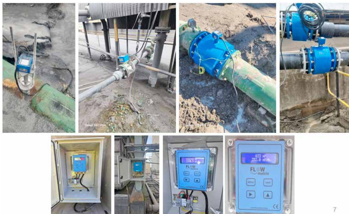
Figure 2: Newly electromagnetic flow meters installed on raw and potable water pipelines
